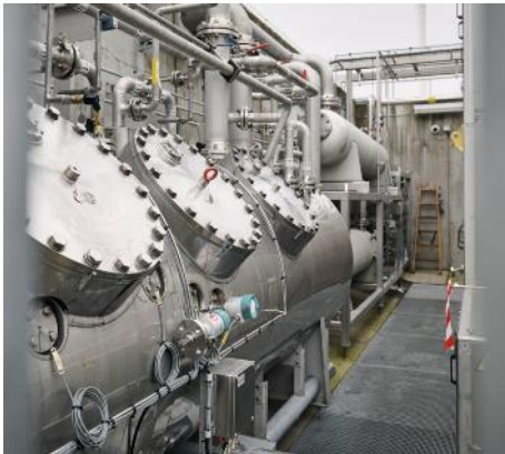
Ammonia catch system
