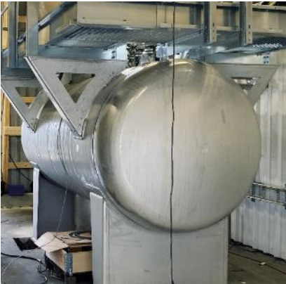
Ammonia service tank
