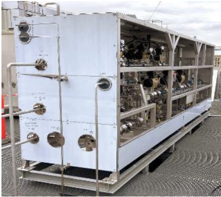
Fuel valve and return train
