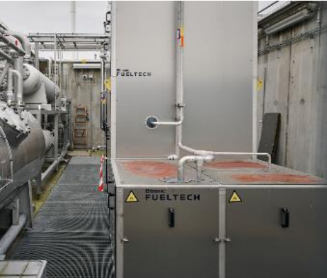
Ammonia supply and recirculation system
